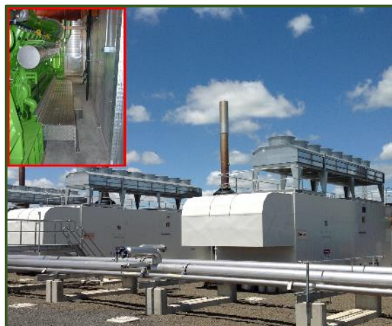
Typical Clarke Energy power station configuration
