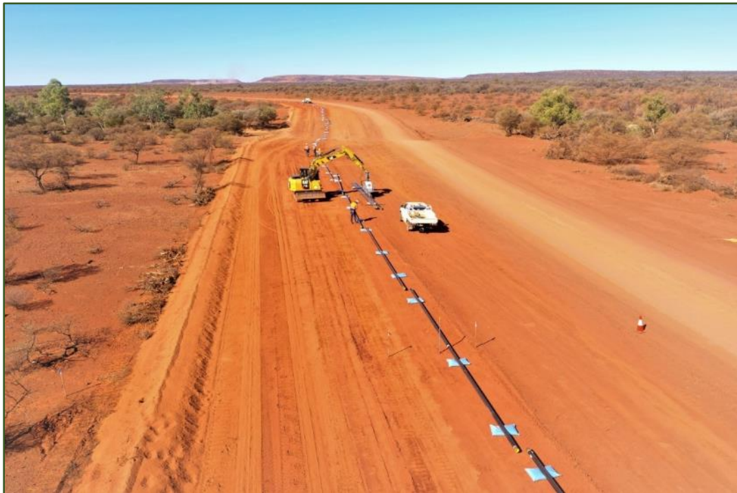
Gas pipe being placed along the access road to the Beyondie SOP Project
