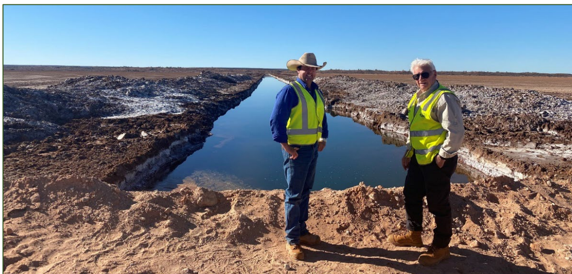
Trenching Works on Sunshine Lake with Director / Founder, Brent Smoothy (left) and Chairman, Mal Randal
